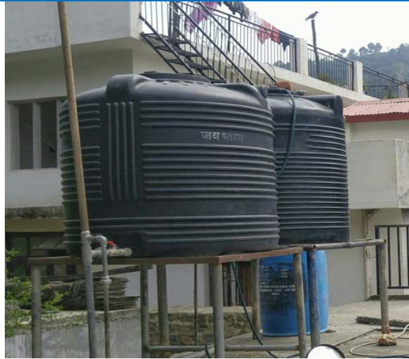
Figure 3: Rooftop Water Storage Tanks in Mandi Town (Photo: J. Agresta)
