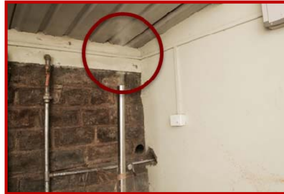
Figure 13. Smoke escaping from top back pipe during testing (Zhang, 2016)
