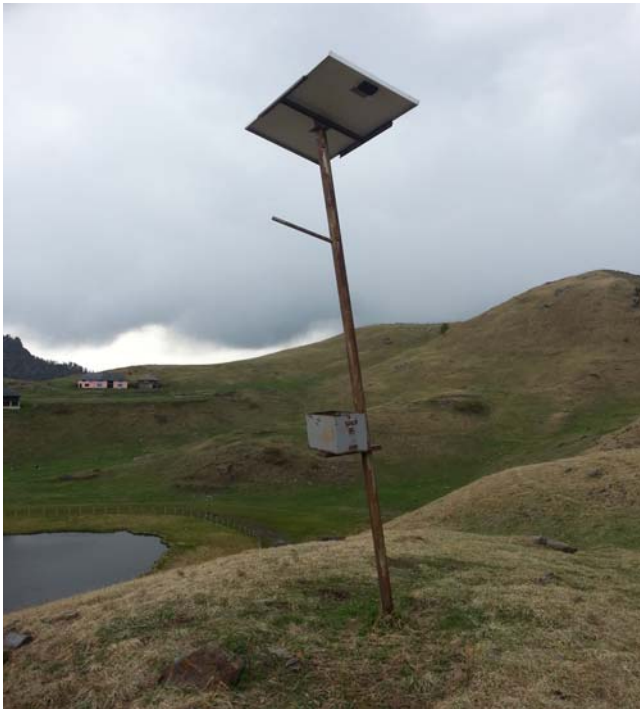
Figure 8. Broken light at Prashar Lake
