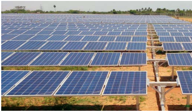
Figure 3. A 4 MW PV installation in Tamil Nadu, India (Wikimedia Commons)
