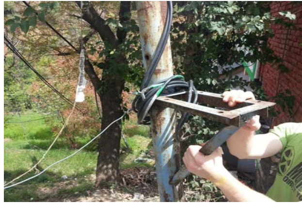
Figure 1. A broken solar street light with a missing battery
